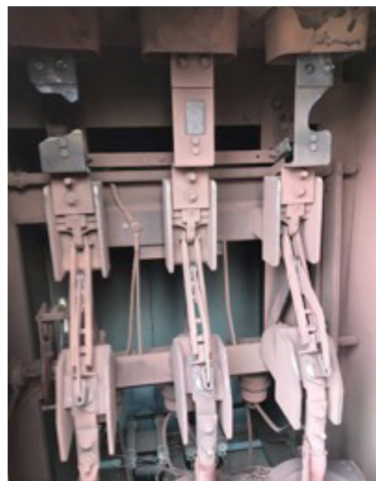
Figure 1 – Image of failed incoming switch
